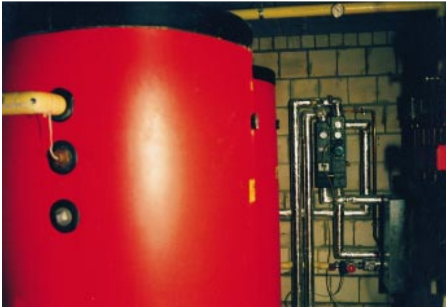
Technikraum Hotel Seenot
